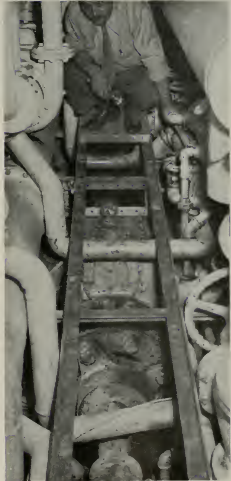
View in shaft alley of Sherry Ann, showing Al Witham inspecting installation of Western Gear planetary reducing set under floor of alley.
